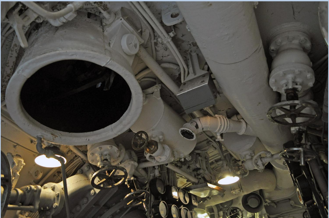
The Main Induction valve was a critical piece of equipment.
